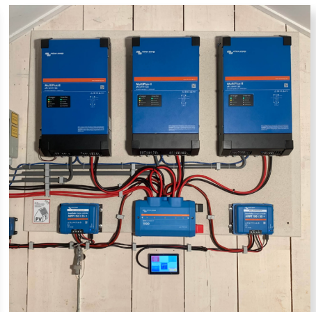
Inverters turnkey installed
