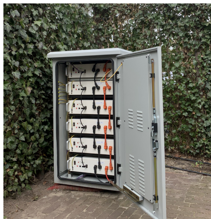
Modular Battery system
